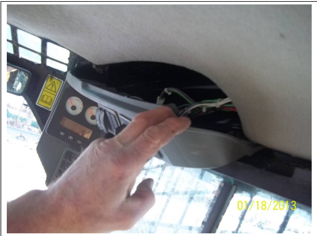
Looking for plug to connect the new switch.
