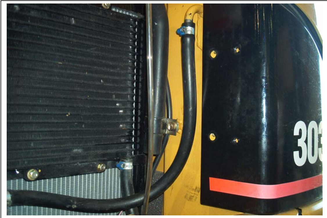
Condenser lower brackets bolts here.
