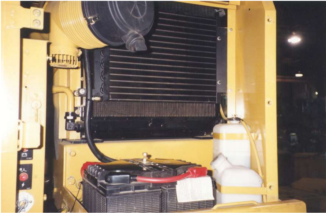
View of condenser in place on radiator.
