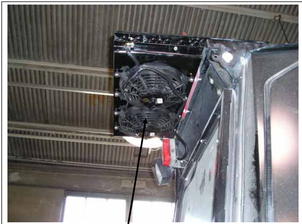
Electric condenser mounted off of back roof of cab.
